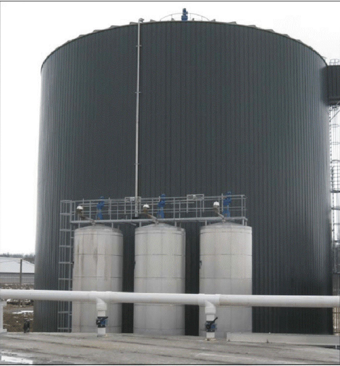
TYPICAL PASTEURISATION TANKS (N.T.S.) (FOREGROUND)
